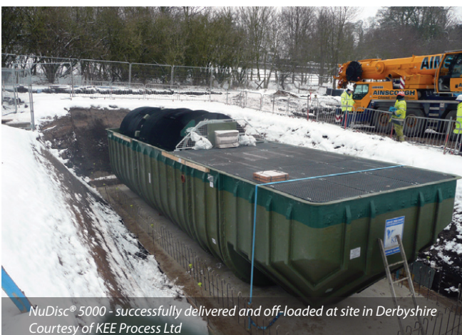
KEE NuDisc® 5000 being offloaded onto concrete slab Courtesy of KEE Process Ltd
