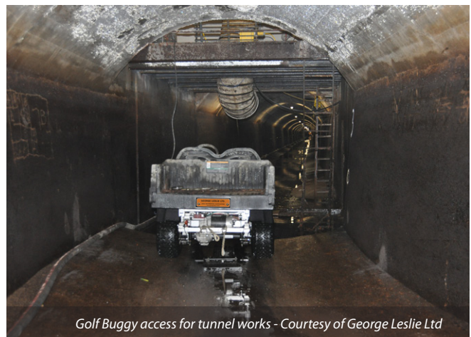
Man-access and tunnel ventilation shaft Courtesy of George Leslie Ltd
