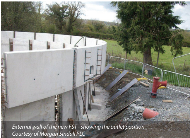
Internal view on the new FST - showing the anti-flotation flap valve positions - Courtesy of Morgan Sindall PLC
