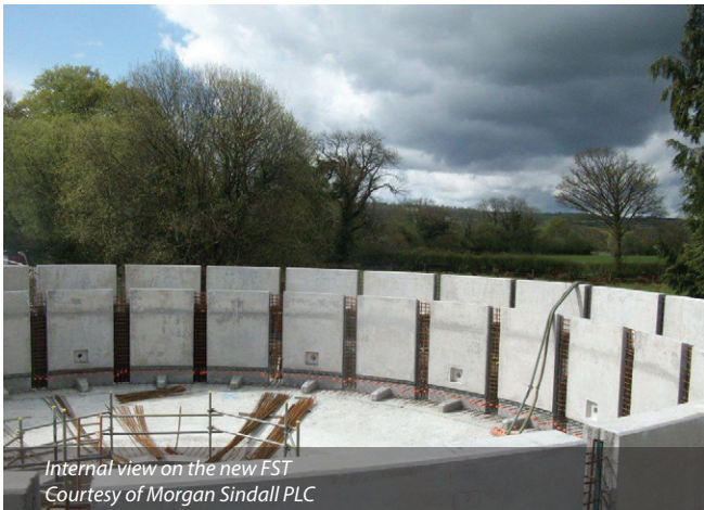
External wall of the new FST - showing the outlet position - Courtesy of Morgan Sindall PLC
