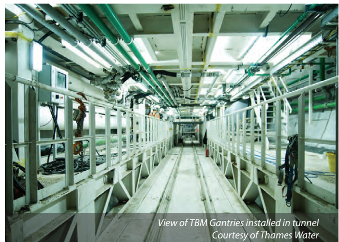
View of the surface of Overflow Shaft showing a TBM Gantry being lifted into launch shaft - Courtesy of Thames Water
