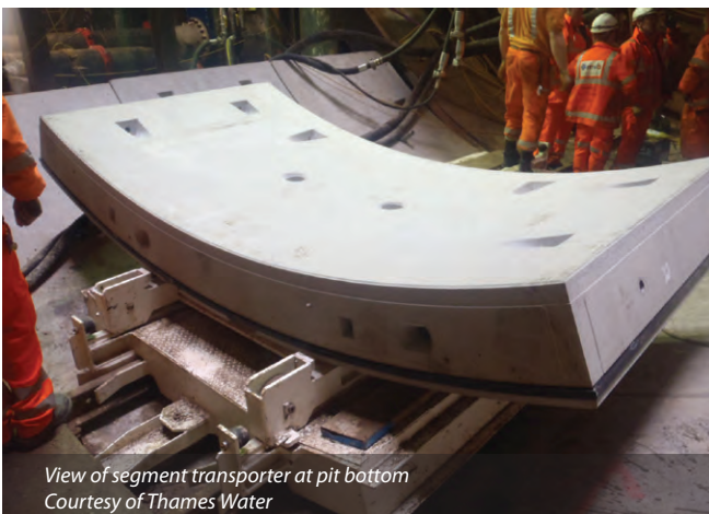
Launch platform set-up complete with TBM control cab and units on the top level - Courtesy of Thames Water
