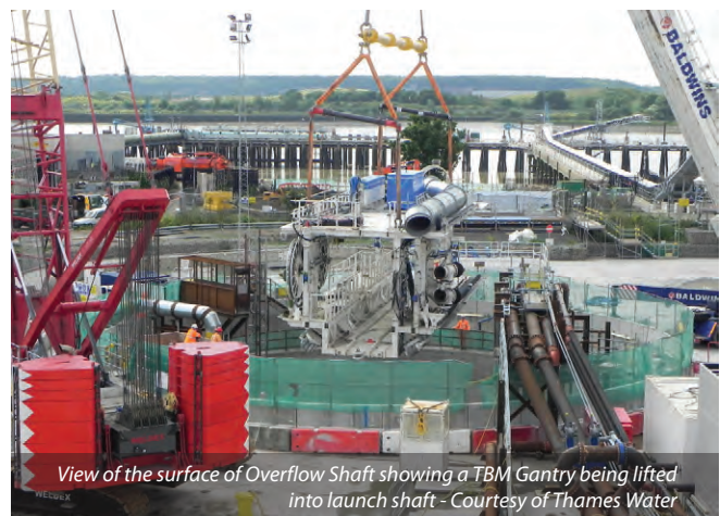
A pre-assembled TBM Gantry being transported to launch site Courtesy of Thames Water
