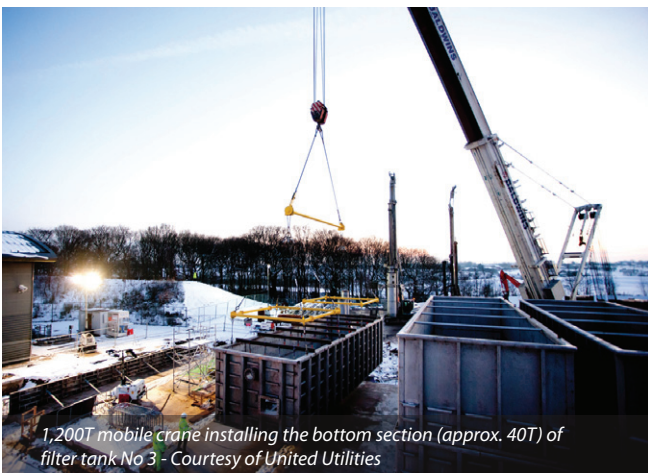
42m concrete pump installing concrete benching to the back wash tank - Courtesy of KMI
