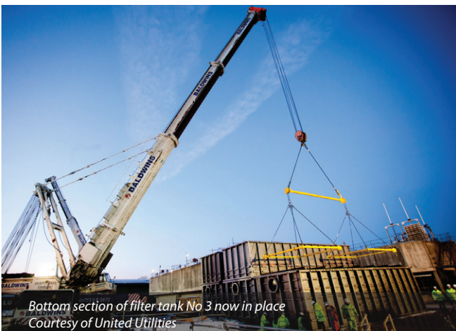
1,200T mobile crane installing the bottom section (approx. 40T) of filter tank No 3 - Courtesy of United Utilities
