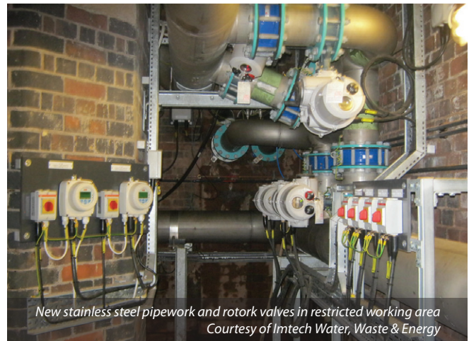
Associated pipework Courtesy of Imtech Water, Waste & Energy
