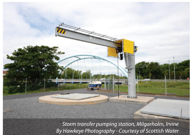
New storm inlet works, Meadowhead Treatment Works, Irvine By Hawkeye Photography - Courtesy of Scottish Water
