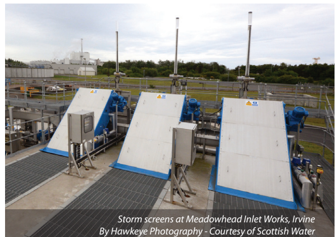
Storm screens and compactor unit at Meadowhead Inlet Works, Irvine By Hawkeye Photography - Courtesy of Scottish Water
