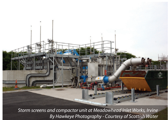
Storm transfer pumping station, Milgarholm, Irvine By Hawkeye Photography - Courtesy of Scottish Water
