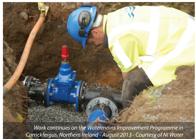
Watermains Improvement Work at the North Road, East Belfast Courtesy of NI Water
