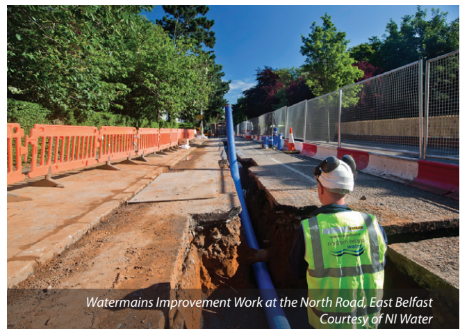
Work continues on the Watermains Improvement Programme in Carrickfergus, Northern Ireland - August 2013 - Courtesy of NI Water
