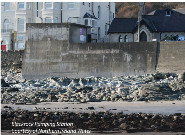
Newcastle: View from existing WwTW towards Blackrock PS and South Promenade - Courtesy of Northern Ireland Water
