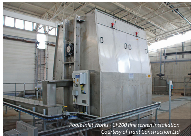
Poole Inlet Works: 3 (No.) Kuhn KWP wash presses Courtesy of Trant Construction
