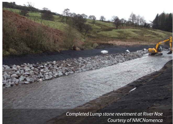
River Noe extraction at weir - Courtesy of Land and Water Services
