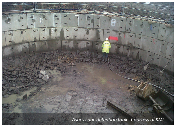
Shaw Road CSO - Courtesy of KMI
