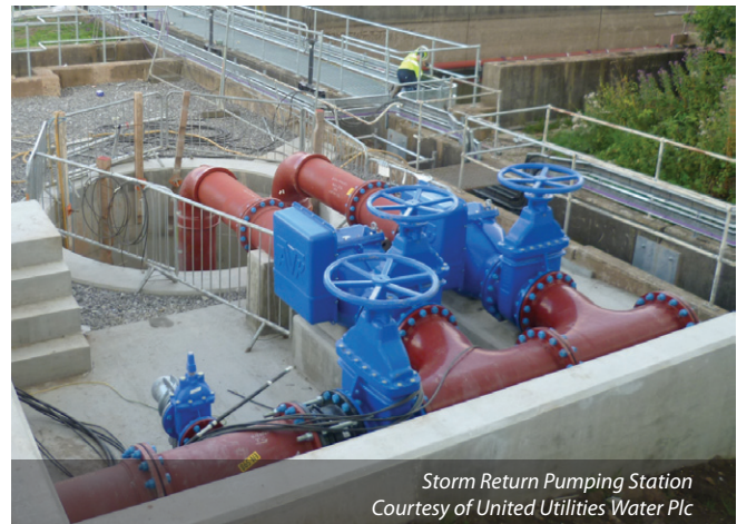
Storm Return Pumping station wet well Courtesy of United Utilities Water Plc
