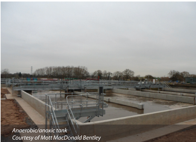
New 4-lane 3-pass ASP lanes with blower kiosk in foreground Courtesy of Mott MacDonald Bentley
