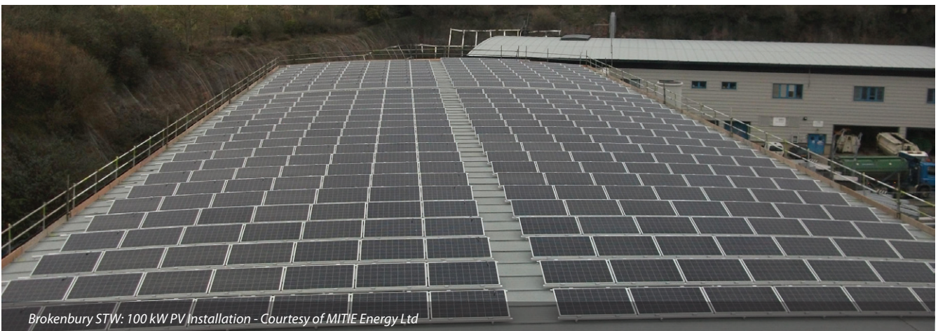
Despite the poor summer of 2012, the forecast generation targets were exceeded
