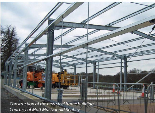
Construction of the new steel frame facility Courtesy of Mott MacDonald Bentley
