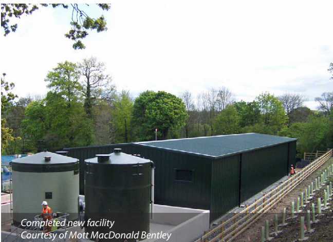
Construction of the new steel frame building Courtesy of Mott MacDonald Bentley
