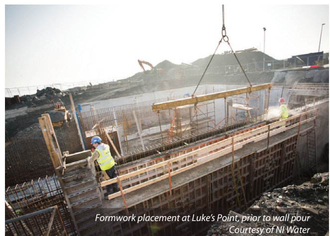
(Right) Wall reinforcement at Luke's Point. (Left) Sheer rockface following excavation - Courtesy of NI Water
