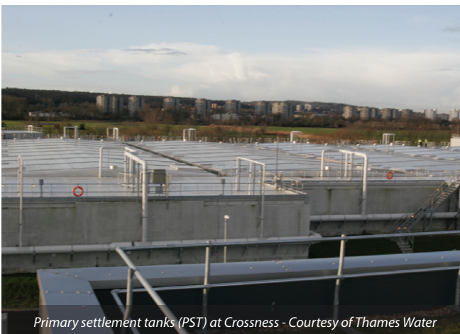
Eastern ASP lane at Crossness - Courtesy of Thames Water
