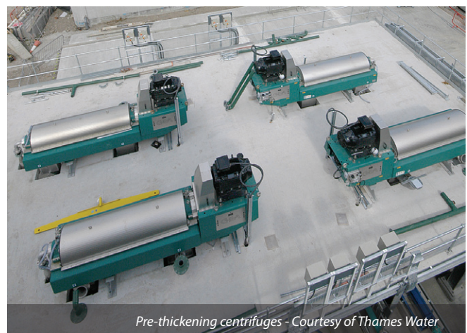
Beckton STW: Bucher final dewatering hall - Courtesy of Thames Water
