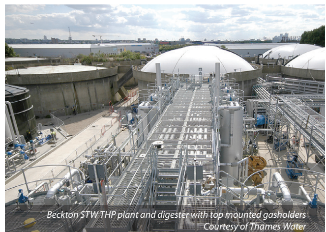
Pre-thickening centrifuges - Courtesy of Thames Water
