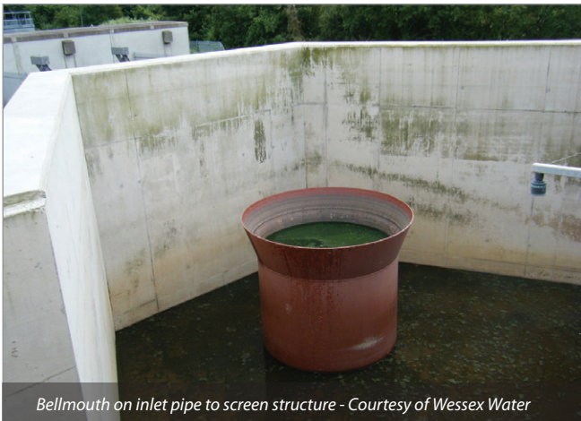
Existing screens overwhelmed - Courtesy of Wessex Water
