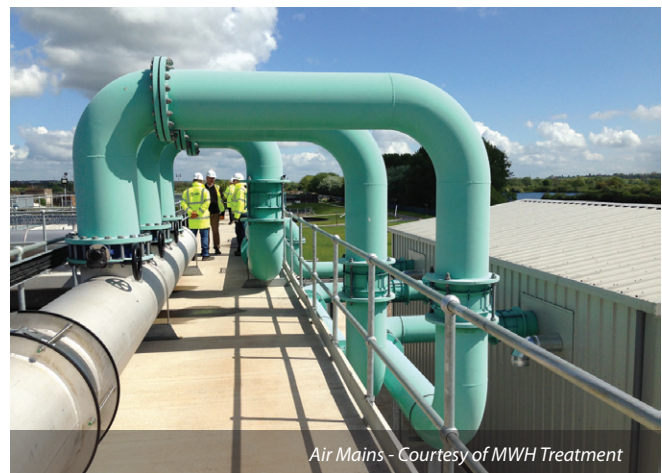
Bio-P carbonaceous ASP - Courtesy of MWH Treatment
