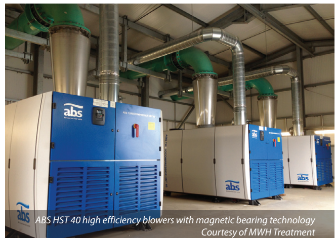
Air Mains - Courtesy of MWH Treatment
