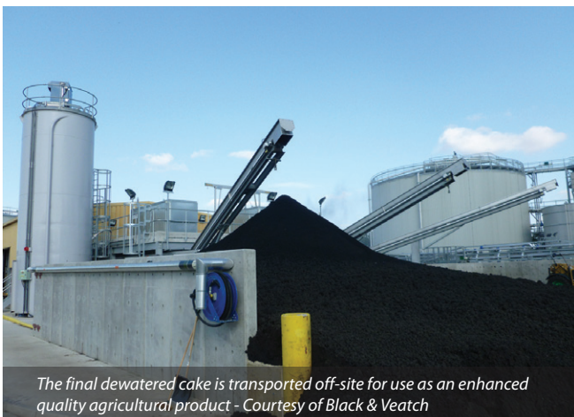
New GBT building (left), cake silo (centre) and cake reception facility (right) - Courtesy of Black & Veatch
