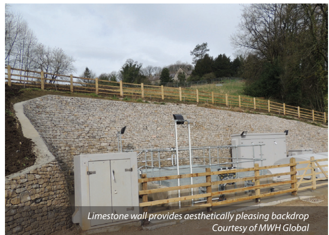
RBC and balance tank - Courtesy of MWH Global
