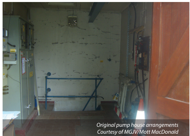
Original below ground dry well - Courtesy of MGJV/Mott MacDonald
