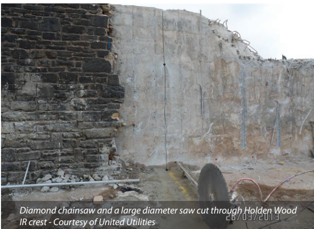
Temporary King Post wall at Holden Wood IR Looking downstream from embankment crest - Courtesy of United Utilities
