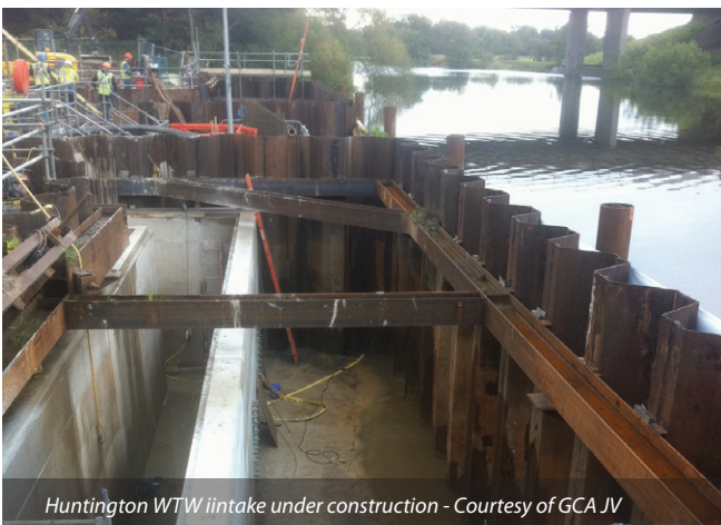
Huntington WTW inlet works - Courtesy of GCA JV
