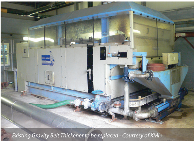
Existing GBT Building, liquors transfer pumping station and odour control unit, all to be modified - Courtesy of KMI+
