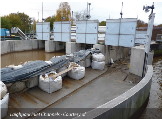
Laighpark STW upgrade - Courtesy of MWH Treatment
