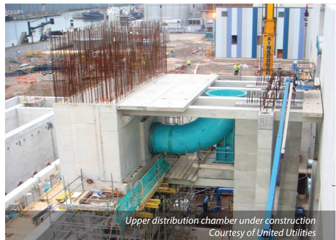
Refurbishment of existing primary settlement tank assets: chain and boom - Courtesy of United Utilities
