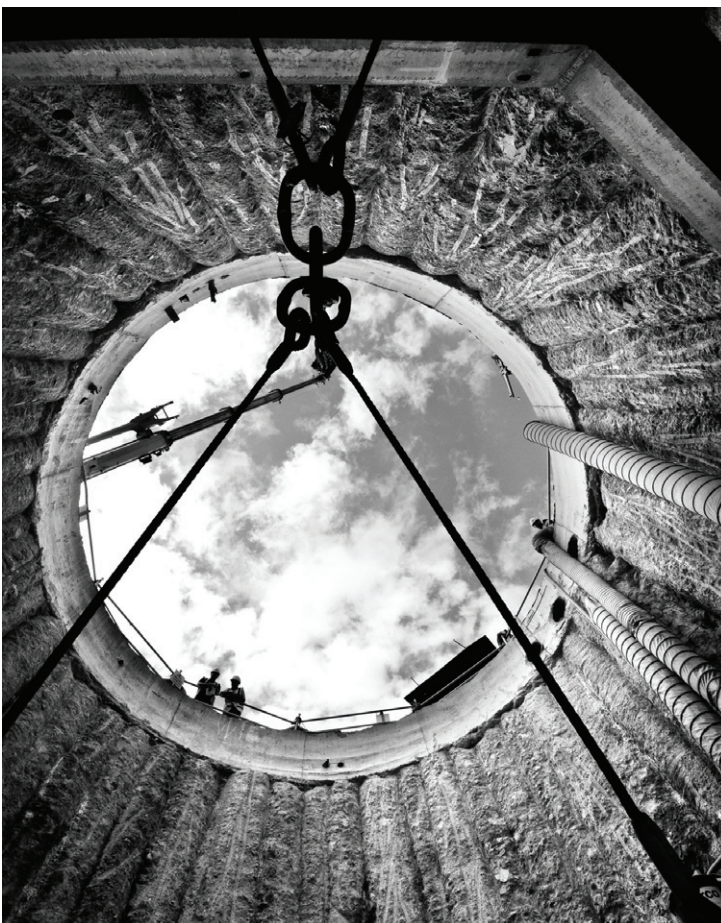
Viewpoint from base level of the Duke Street WwPS scheme shaft showing the secant pile construction method employed - Courtesy of AECOM Ltd
