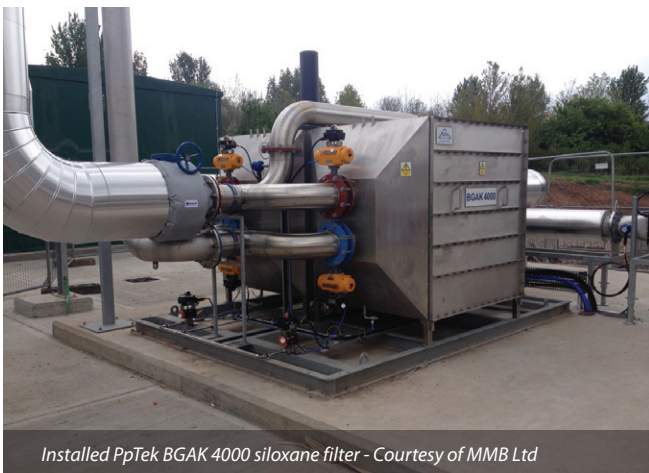
CHP installation complete and commissioning underway Courtesy of MMB Ltd
