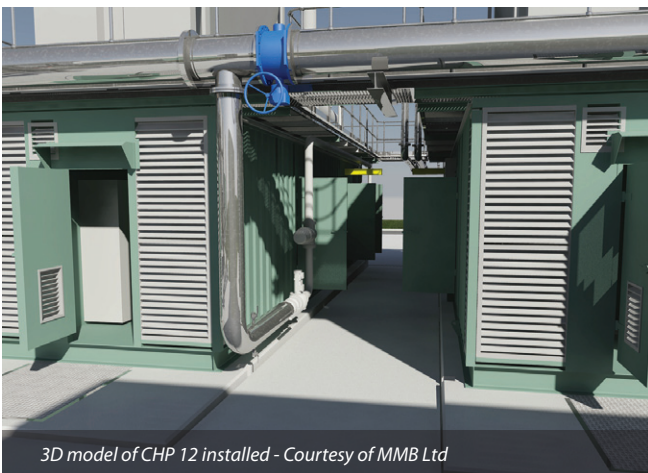
CHPs 10, 11 and 12 with process water pipework suspended from cantilevered access platform - Courtesy of MMB Ltd
