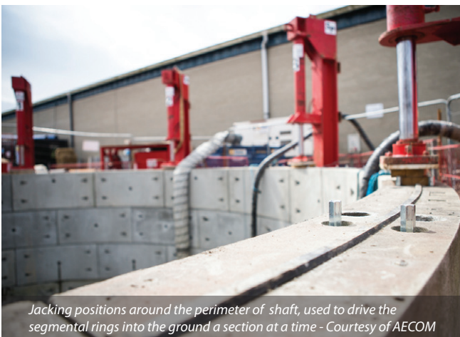
Overlooking the foul and stormwater wet wells, illustrating the complexity of the caisson construction - Courtesy of AECOM Ltd
