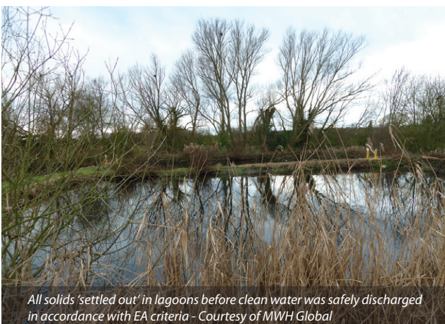
Groundwater constantly pumped from excavation to a series of settlement tanks in one of the wettest periods on record Courtesy of MWH Global
