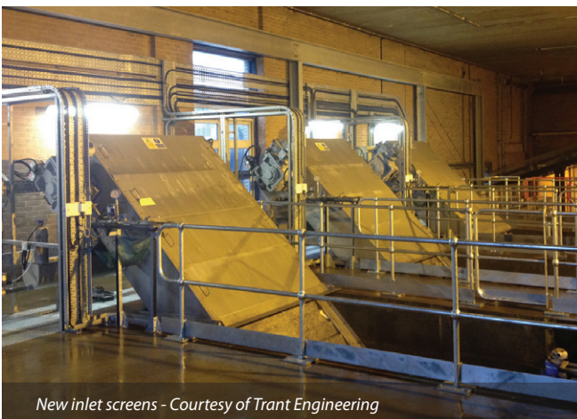
MCC - Courtesy of Trant Engineering
