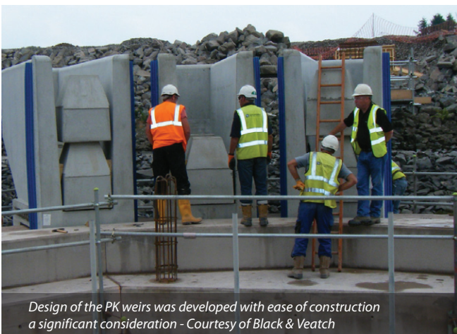
Working over water was minimised, most construction occurred on the original bellmouth rim, around which temporary working platforms were deployed - Courtesy of Black & Veatch
