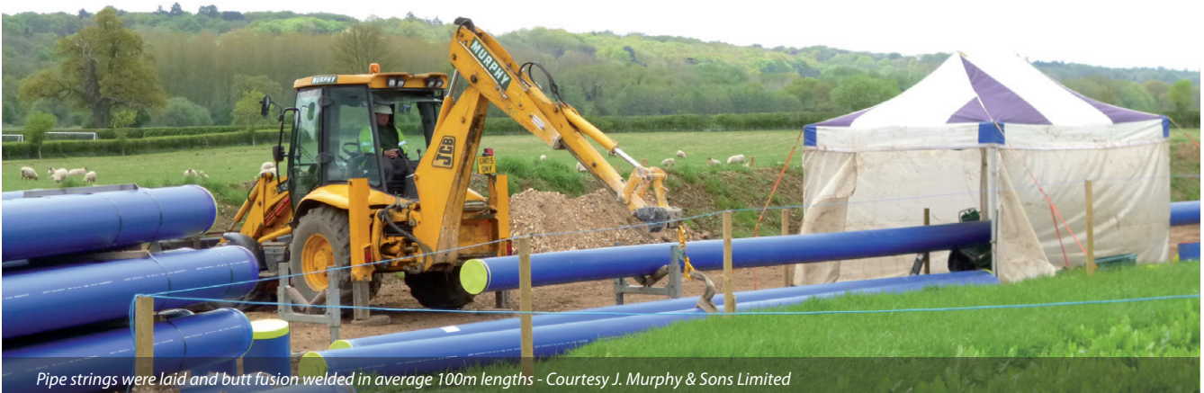
The pipeline emerges from a directional drilling pit Courtesy J. Murphy & Sons Limited
