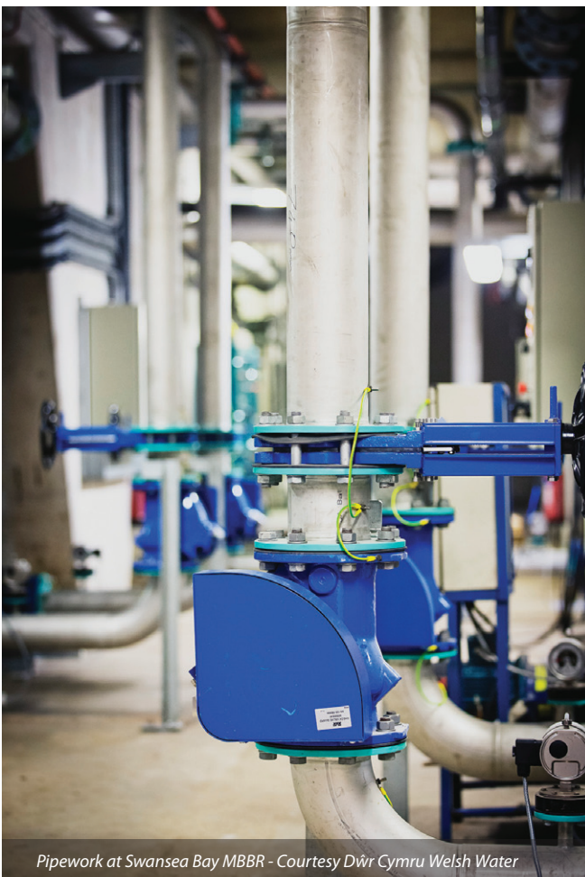
Process Plant at Swansea Bay MBBR - Courtesy Dŵr Cymru Welsh Water
