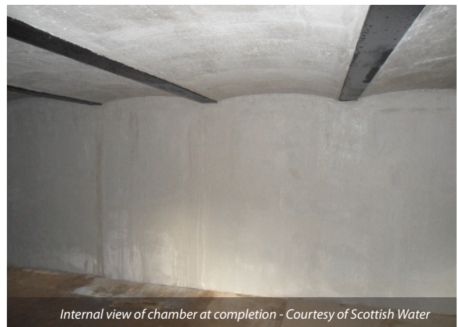
Overflow chamber - pile cap - Courtesy of Scottish Water
