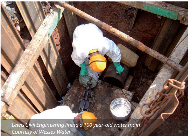
The extent of the corrosion in an ageing iron main Courtesy of Wessex Water
