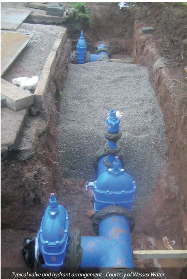
Lewis Civil Engineering lining a 100 year-old water main Courtesy of Wessex Water
