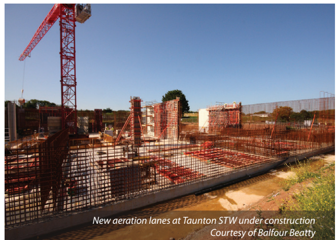
Final settlement tank - Courtesy of Balfour Beatty
