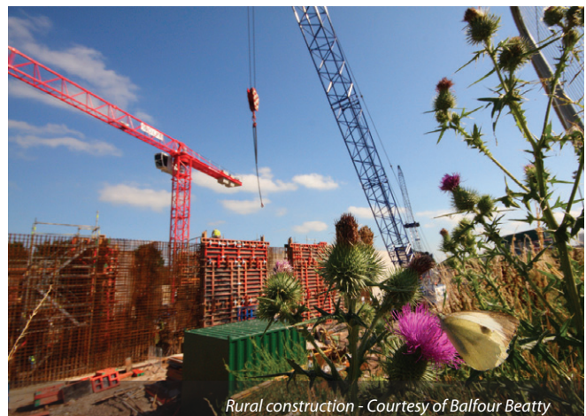
New aeration lanes at Taunton STW under construction Courtesy of Balfour Beatty
