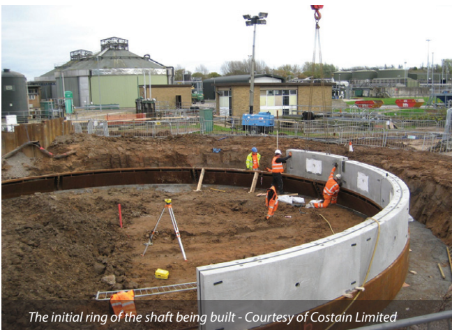
The shaft for the storm pumping station under construction Courtesy of Costain Limited
