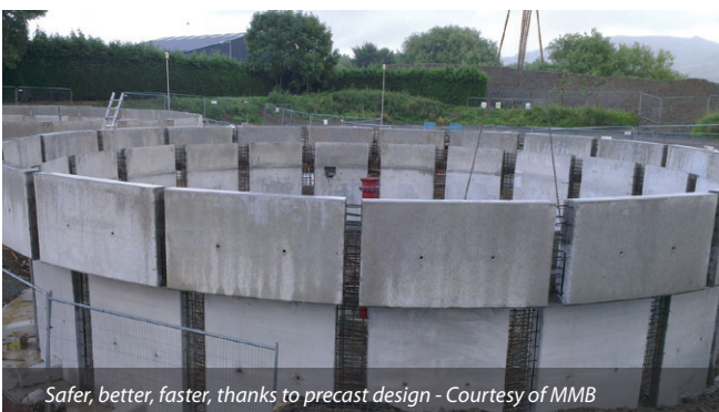
One of the 13.5m diameter final settlement tanks with half bridge scrapers - Courtesy of MMB
