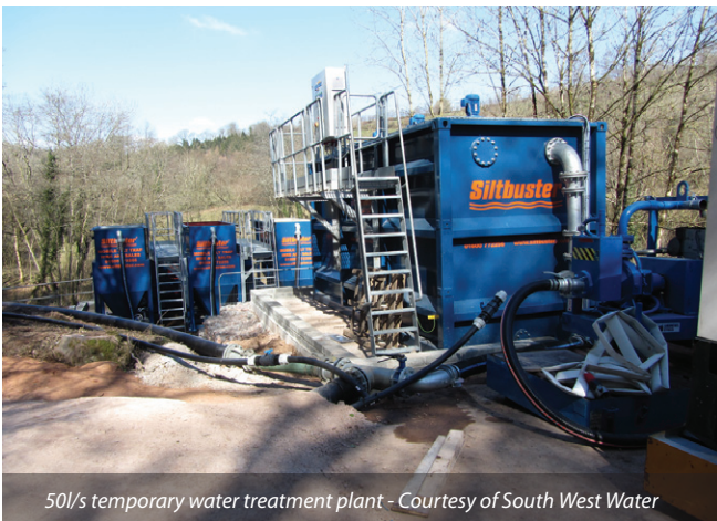
50l/s temporary water treatment plant Courtesy of Chris Mills, Still Imaging
