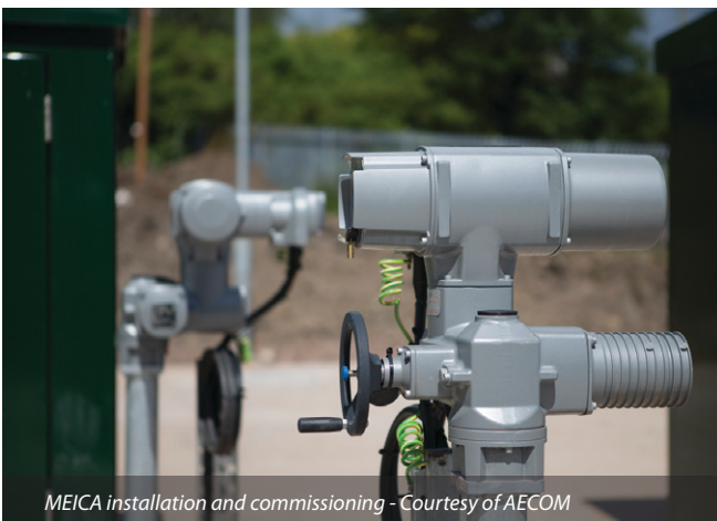
Staged-lift pumping station internal Courtesy of AECOM
