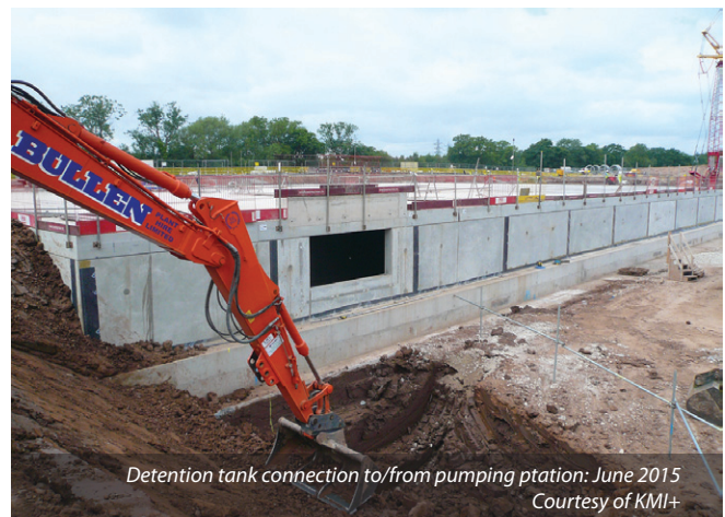
Flushing chambers 1 of 2 connecting orifices: May 2015 Courtesy of KMI+
