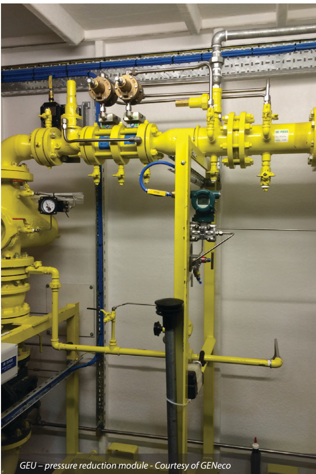
GEU – propane injection assembly - Courtesy of GENeco
