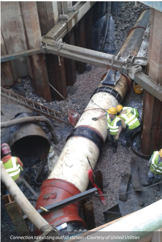
Connection manifold at pumping station - Courtesy of United Utilities
