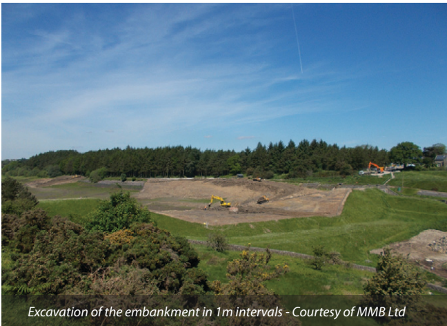
View of the upstream face of the dam before commencement of works Courtesy of MMB Ltd
