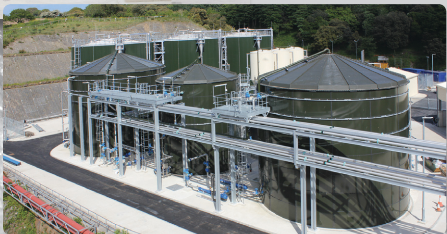
Sludge storage tank Courtesy of the States of Jersey
