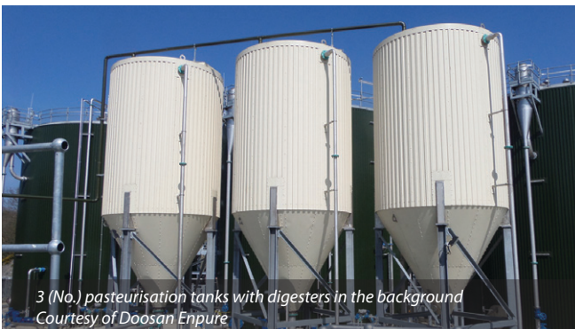
View from cake store prior to road completion Courtesy of Doosan Enpure
