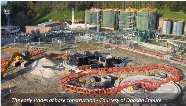
Pasteurisation & anaerobic digestion plant - Courtesy the States of Jersey
