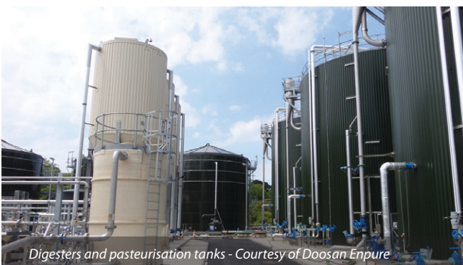
3 (No.) pasteurisation tanks with digesters in the background Courtesy of Doosan Enpure
