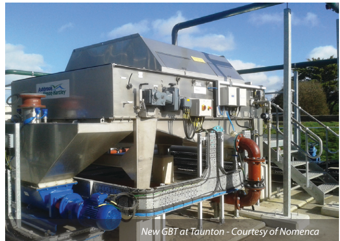
New Digester at Taunton STW - Courtesy of Nomenca
